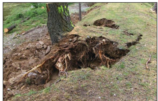
Figure 13. Dike degradation due to a falling pine tree (Source: CZ)
