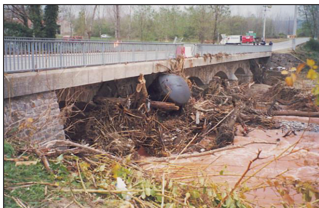
Figure 11. Bridge obstruction by log-jams (Source: www.aquadoc.fr -1999 flood on Thoré river)
