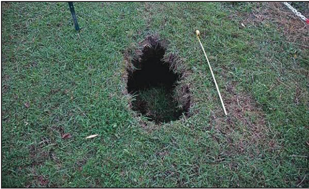
Figure 14. Sinkhole induced by stump decomposition and generating risk of internal erosion (Source: PM)
