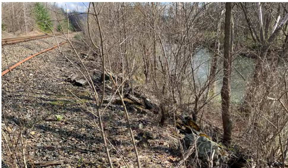
In one short section, the river is close to the rail berm.
