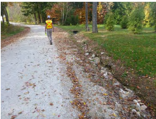
Photo 1: Severe erosion of undersized ditch leading to cross-culvert.
