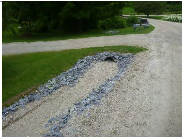
Photo 2: Check dams and a sediment trap along Prouty Hill road are filled with sediment from ditch and road erosion.
