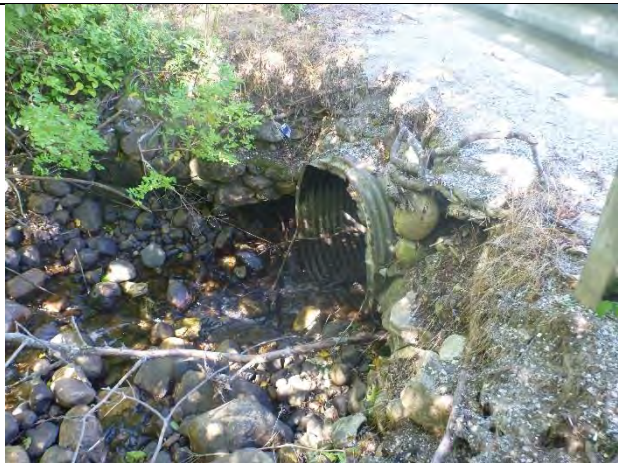
Photo 1: An undersized culvert under Sunderland Hill Road, with a steep embankment and erosion at the inlet.
