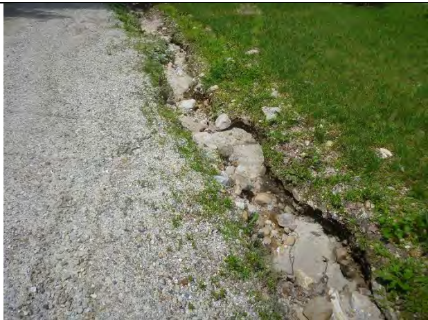
Photo 1: Eroded undersized ditch along Barney Orchard Rd.
