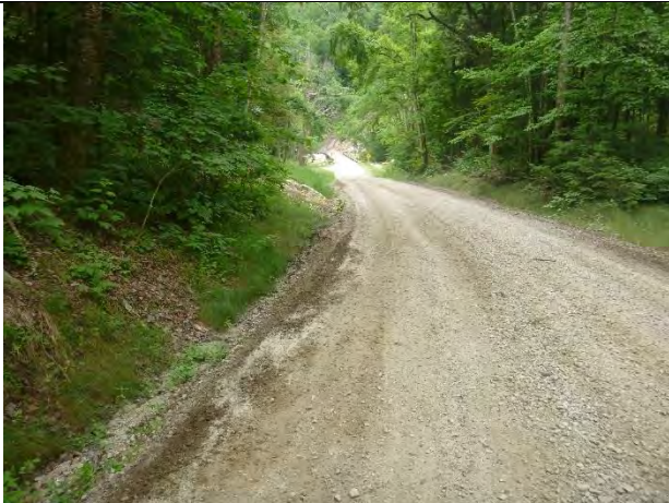
Photo 1: A steep eroding ditch along Kelley Stand Road.
