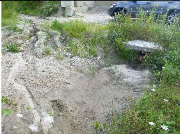
Photo 1: A sediment trap along Dunham Road that the Town sand pit and salt shed area drains to.
