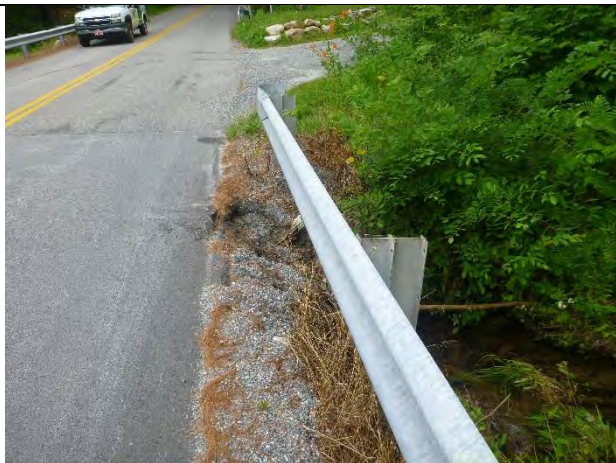
Photo 1: A culvert under North Road is too short causing erosion of the road shoulder at the culvert inlet.
