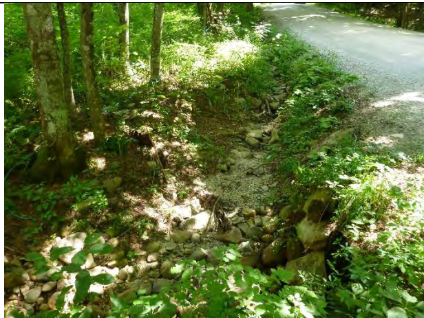
Photo 2: Incised ditch at the stream crossing is delivering large volumes of sediment and gravel.
