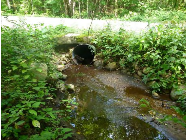
Figure 2: Sand and gravel deposition in the channel upstream of the culvert inlet.
