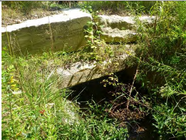
Photo 1: Location of a collapsed inlet to a cross culvert under South Road.
