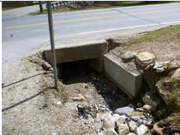
Photo 2: Inlet of the undersized box culvert at Route 7a
