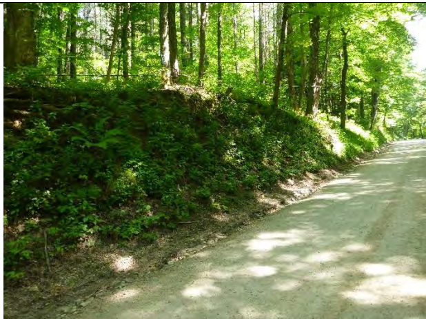
Photo 1: Poorly defined ditch with gully erosion along Laver Road.
