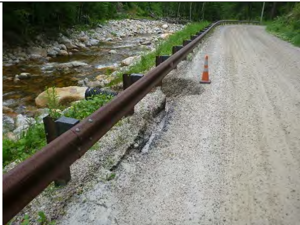
Photo 1: Gully erosion along Kelley Stand Road.
