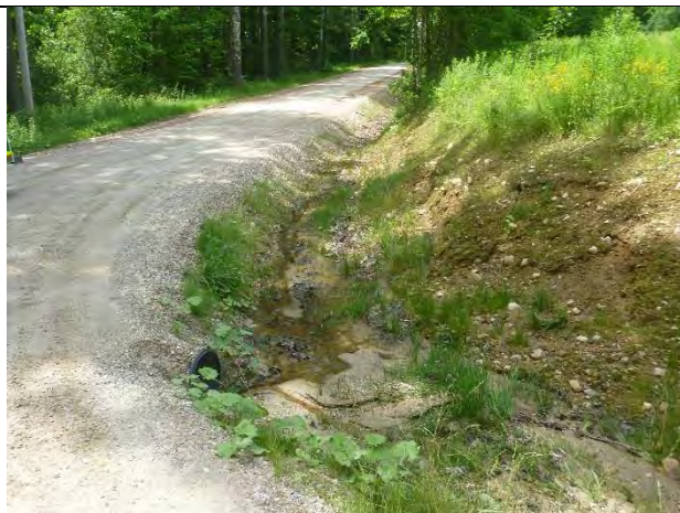
Photo 2: Sediment at the inlet of the culvert under Flynn Hollow Road.
