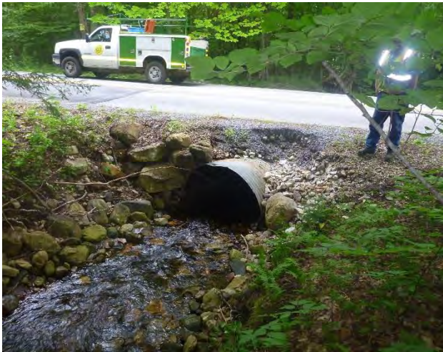
Figure 1: Embankment erosion at the culvert inlet.
