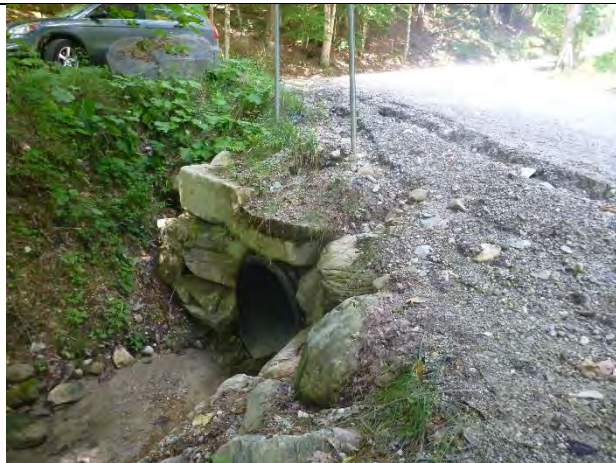
Photo 2: Sediment deposits at the stream culvert outlet from severe gully erosion along the road.
