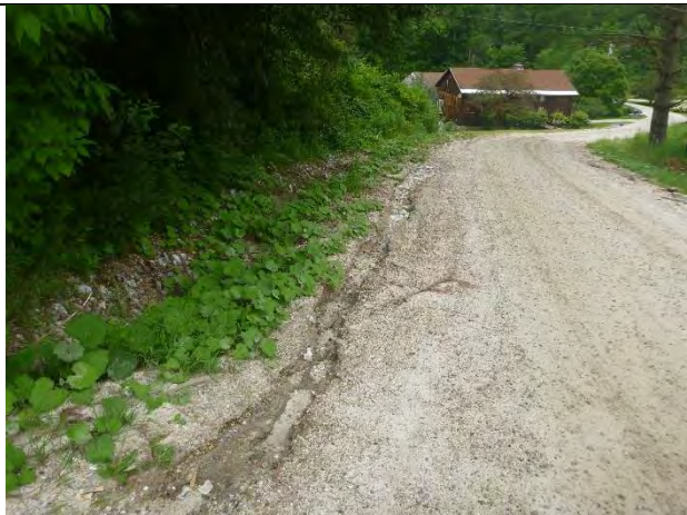
Photo 1: Road erosion along Prouty Hill Road.
