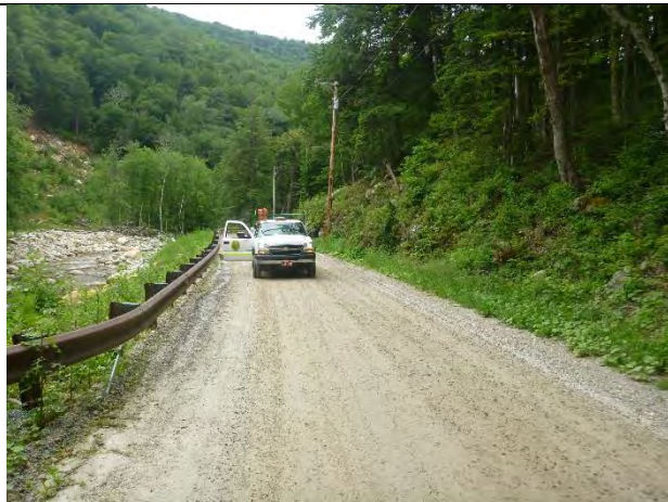
Photo 2: Erosion along the road delivers sediment to the adjacent river.
