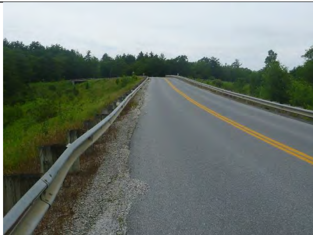
Photo 2: A section of North Road with active erosion is a sediment source to Beaver Meadow Brook.
