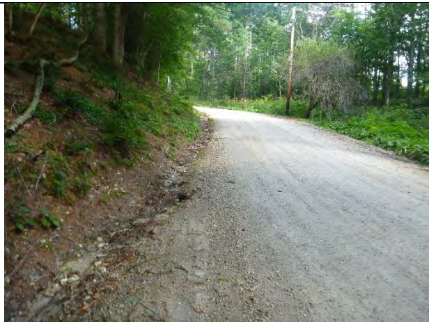
Photo 2: Erosion along Bentley Hill Road, where ditches are shallow and undersized.
