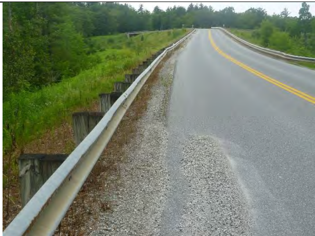
Photo 1: A section of North Road with no ditch.
