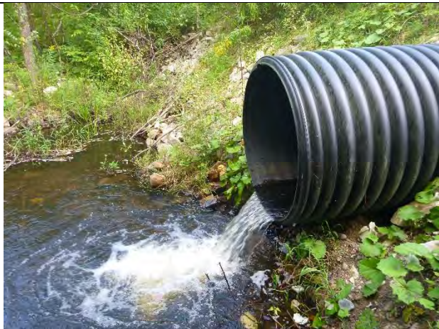
Photo 1: The culvert under South Road is perched.
