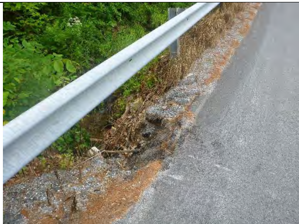
Photo 2: Erosion along the road shoulder due to the vertical banks at the culvert outlet.
