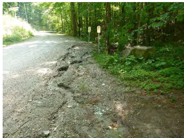
Photo 1: Severe erosion along Bentley Hill Road at the stream crossing location where the ditch spills onto the road at the private driveway.
