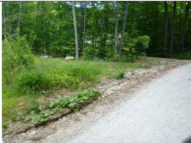
Photo 2: Gully erosion along a section of Shady Pines Road with no ditch.
