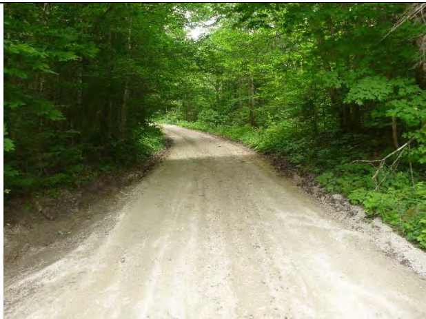
Photo 1: A steep section of Kelley Stand Road, with some active erosion in roadside ditches.
