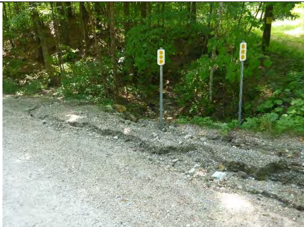
Photo 1: Major gully erosion along Bentley Hill Road.
