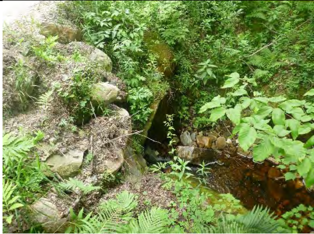
Photo 1: A culvert under Kelley Stand Road is short with near vertical embankments.
