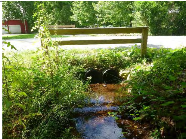
Photo 2: Replacing the culverts with a larger culvert or box and increasing the culvert slope would improve conveyance.
