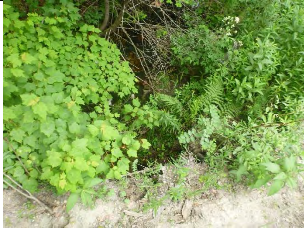
Photo 2: Vertical embankments at the culvert along Kelley Stand Road are prone to erosion.
