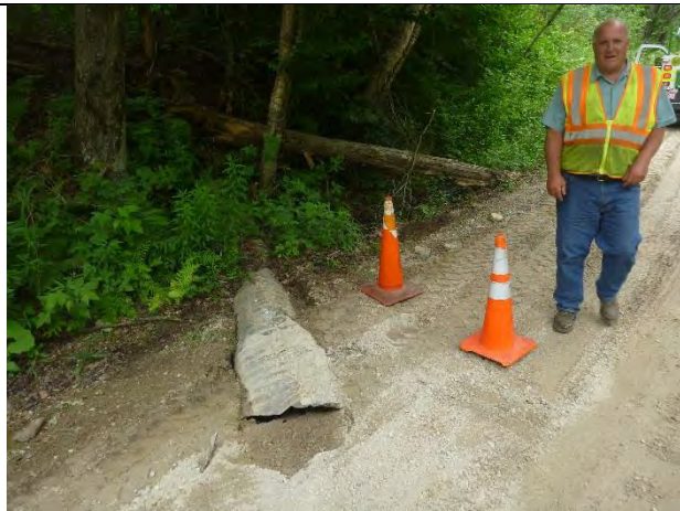
Photo 2: The culvert inlet is damaged and exposed.
