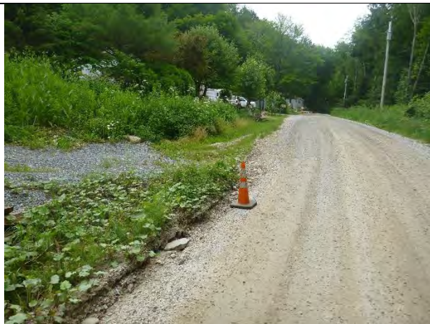
Photo 2: The poorly aligned culvert is interrupting flow and causing erosion along the road and ditch.
