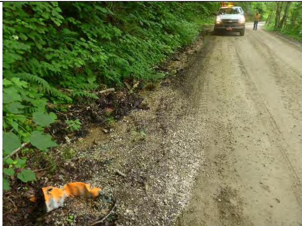
Photo 1: Exposed and damaged cross culverts on Kelley Stand Road.
