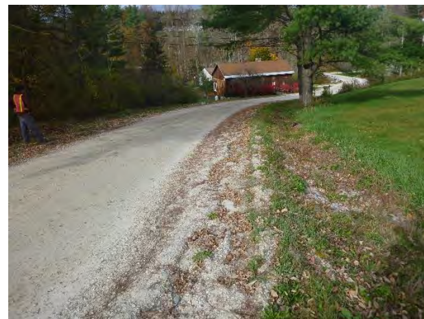
Photo 2: Severe erosion along the road edge where a small grader berm is preventing sheet flow into the ditch.
