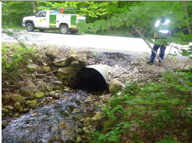
Photo 1: An undersized culvert conveys Cole Brook under North Road.
