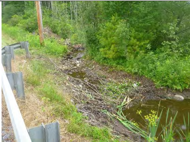
Photo 1: The culvert under Bacon Hollow Road is backwatered.
