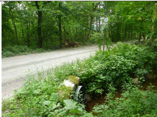
Photo 2: Dunham road washed out in Tropical Storm Irene.
