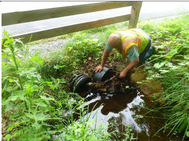
Photo 1: Double culverts under North Road trap sediment, debris and ice.
