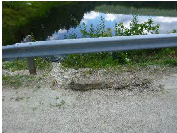
Photo 2: Erosion along the edge of South Road at the culvert outlet.
