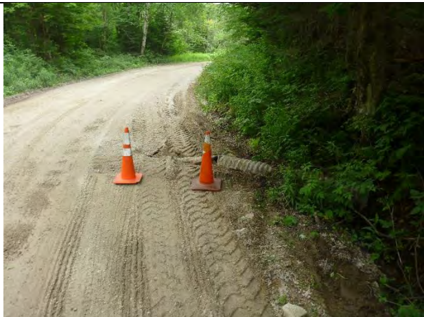
Photo 1: Location of a damaged cross culvert along Kelley Stand Road.
