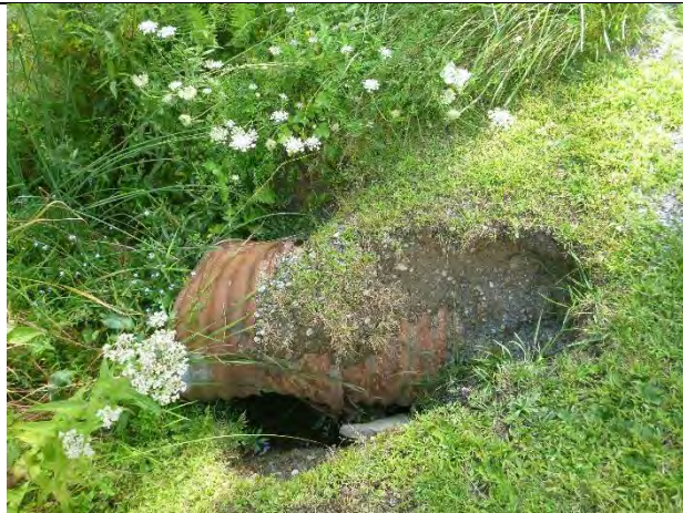
Photo 2: Erosion at the outlet of a cross culvert under South Road.
