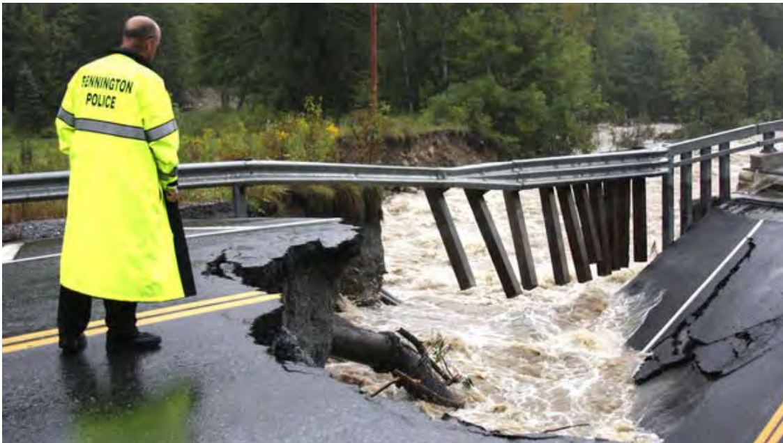
Preventative actions and emergency response preparedness can help mitigate the impact of flood events such as the one pictured above, which compromised a transportation corridor in Bennington (photo from cbsnews.com).
