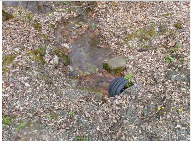
Photo 2: Broken Snow Road cross culvert outlet.
