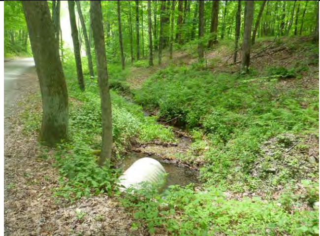
Photo 2: Some bank erosion is present downstream of an undersized culvert on Rupert Road.
