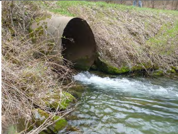
Photo 1: Outlet drop from Baldwin Brook culvert at West Sandgate Road.
