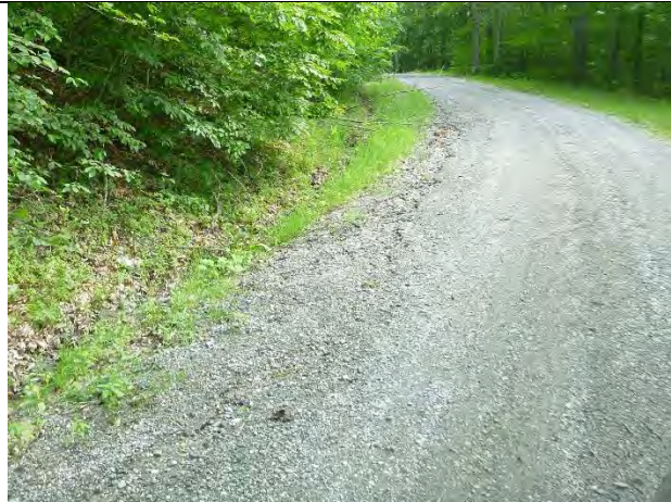
Photo 2: Road erosion along a steep section of Chunks Brook Road.
