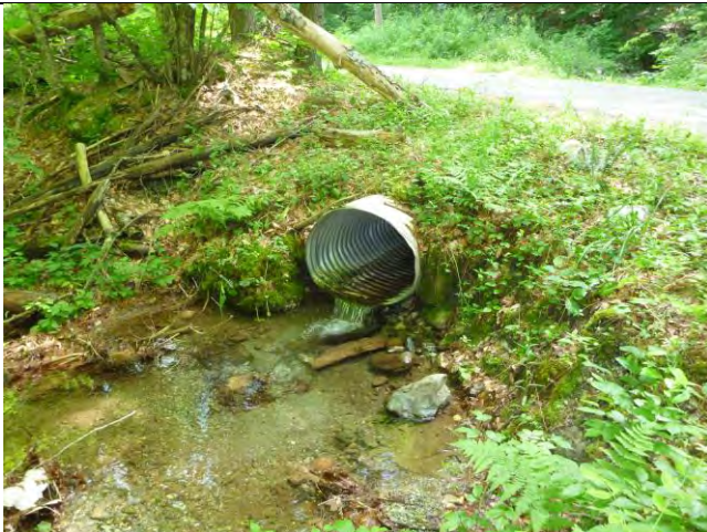
Photo 1: An undersized culvert on Chunks Brook Road.
