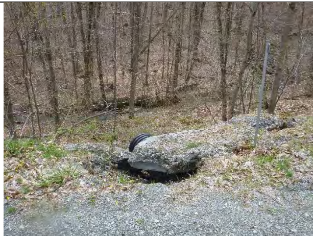
Photo 1: Severe road erosion around the headwall of a cross-culvert outlet on Wilcox Hollow Road.
