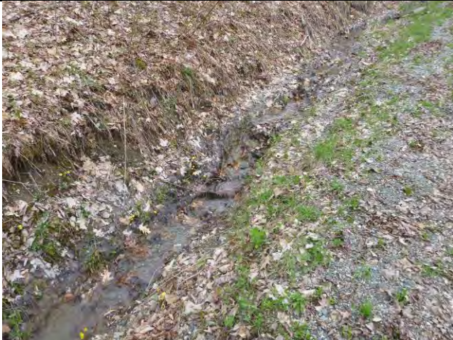
Photo 1: A headcut and erosion in the ditch upstream of a West Road cross culvert.
