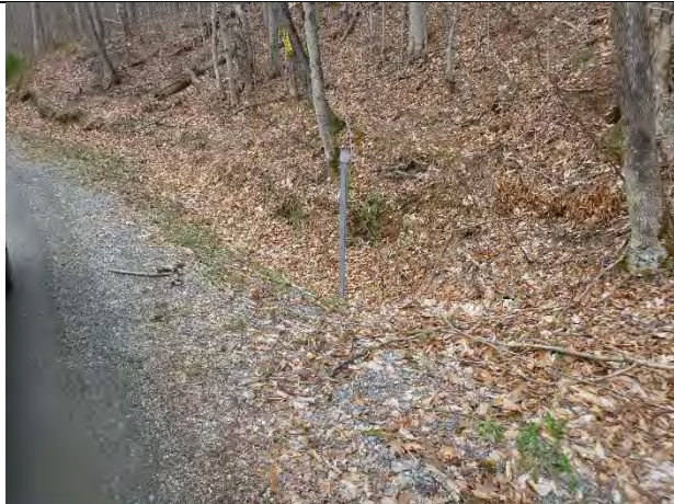
Photo 1: Ditch upstream of cross-culvert inlet on Wilcox Hollow Road is filled in, causing water to follow the road.
