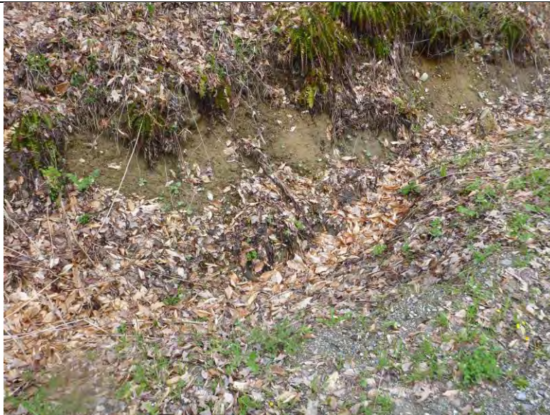
Photo 1: Erosion and a headcut in the Rupert Road ditch upstream of a cross culvert inlet.
