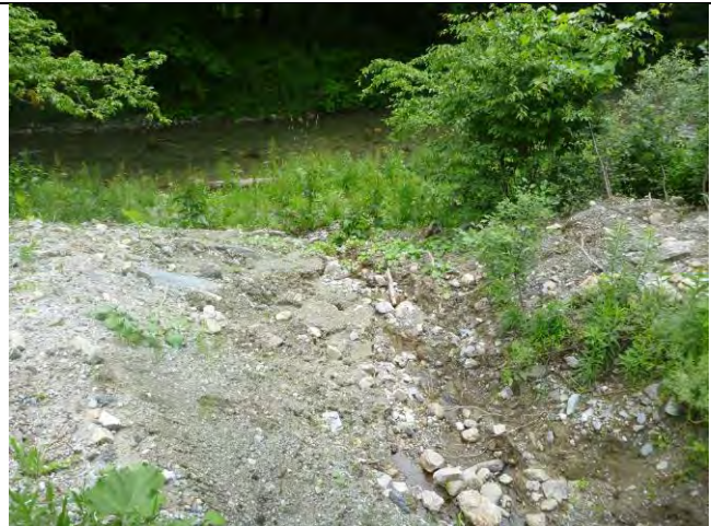
Photo 2: Erosion at a Sandgate Road cross culvert outlet is acting as a source of sediment to the Green River directly downstream.
