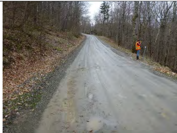
Photo 2: Road grade conveying runoff toward the steep slope and brook, rather than the existing ditch and cross-culvert.
