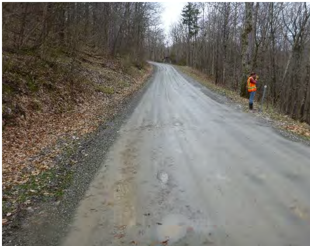
Figure 2: The road crown does not direct water into the existing ditch and cross culvert along a section of Rupert Road.
