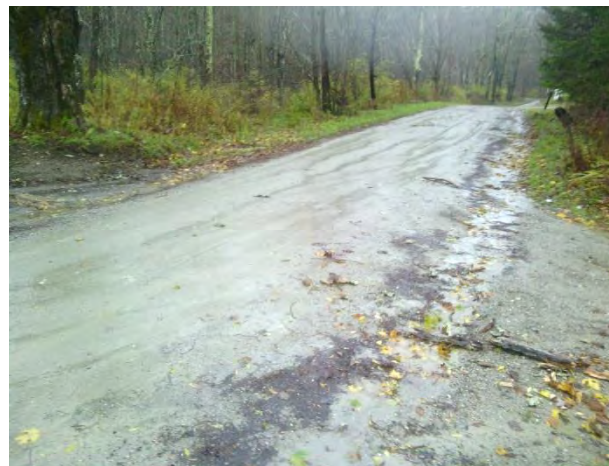
Photo 2: Lower section of Sandgate Road. Runoff is running along the road edge causing rilling and sedimentation downhill.
