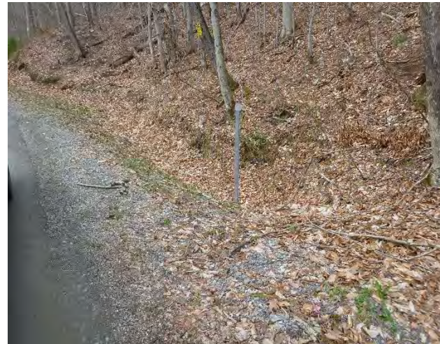
Figure 3: Filling in of the ditch upstream of the culvert may be causing water to spill out of the ditch onto the roadway.
