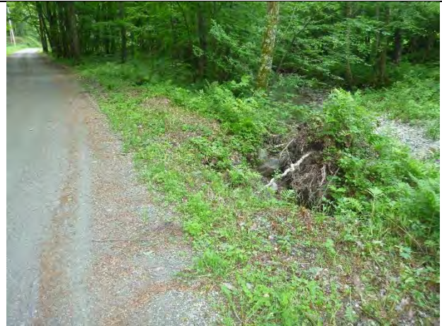
Photo 2: Exposed embankment along Chunks Brook road.
