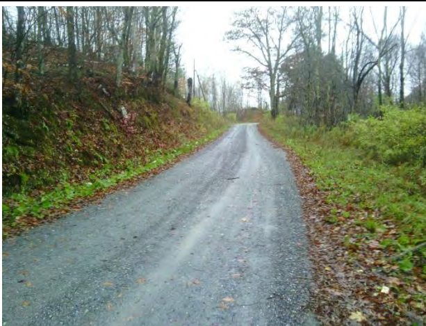
Photo 1: Steep section of upper Wuerslin Road needing stone in ditches and additional cross culverts.
