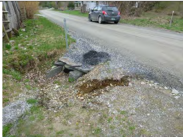
Photo 2: Filled in, poorly defined ditch with erosion where runoff flows along the road over the culvert inlet.
