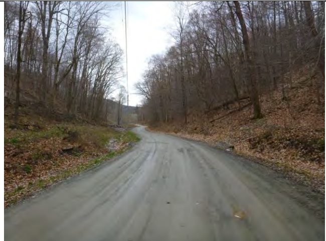
Photo 2: Ditches along a section of Rupert Road are poorly formed and eroding.
