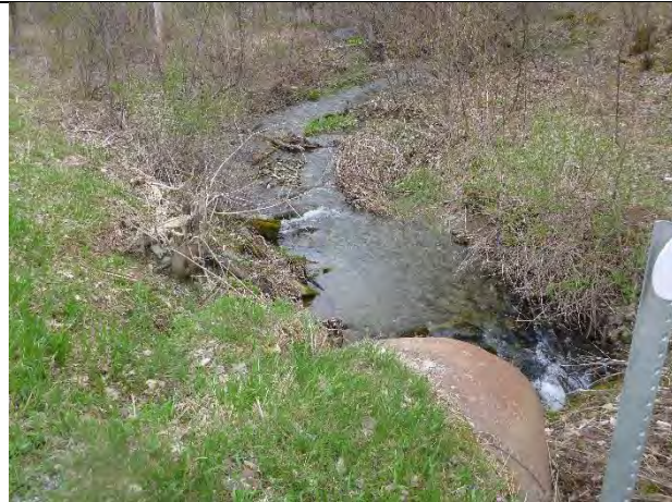
Photo 2: View of downstream channel from roadway. Location of proposed boulder veins to raise tailwater control.
