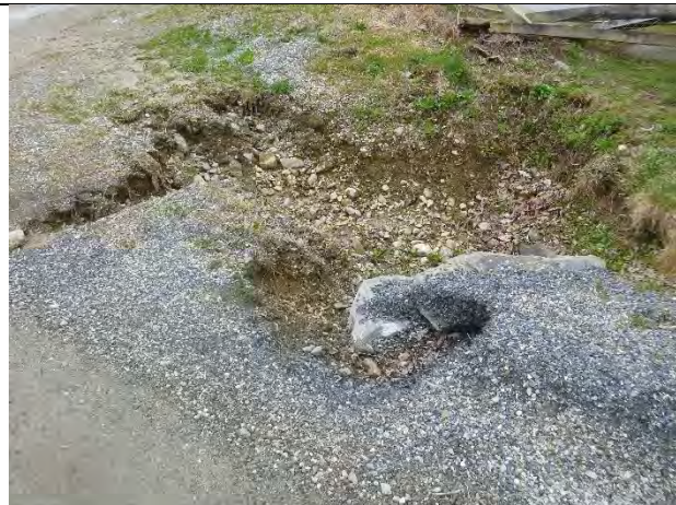
Photo 1: Severe gully erosion along the road edge and at the cross-culvert inlet.
