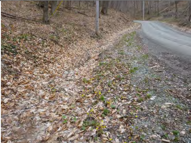
Photo 1: The road crown on a section of Rupert Road is not effectively directing water into the roadside ditches.
