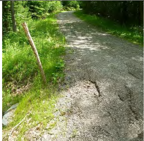
Photo 1: Road erosion to a conveyance at a Chunks Brook stream crossing.
