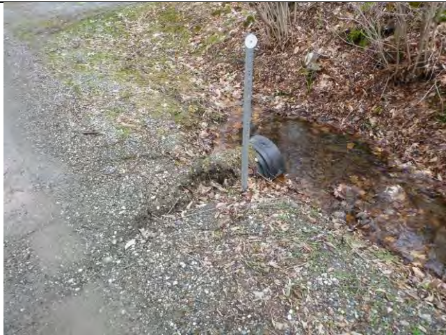
Photo 1: Erosion at the inlet of a Snow Road cross culvert.
