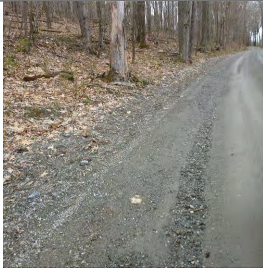
Photo 1: Rill erosion along the side of West Road.
