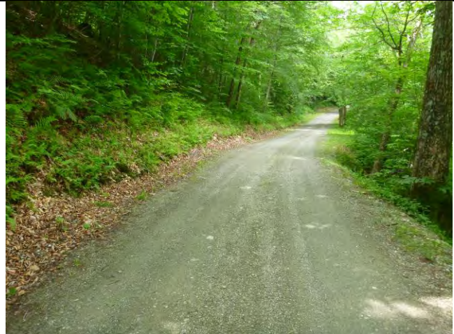
Photo 2: Water currently flowing over the road and eroding the road embankment may be directed into a ditch constructed on the opposite side of the roadway.
