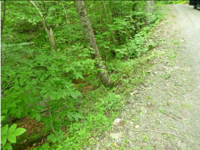
Photo 1: Erosion of a steep road embankment along Tate Hill Road.
