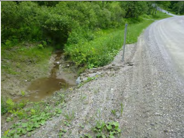
Photo 1: Water flowing over Sandgate Road is causing erosion at a cross culvert inlet, acting as a source of sediment to a roadside wetland.
