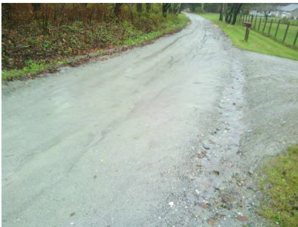
Photo 1: Upper section of Sandgate Road at Woods Gift Lane. Runoff is running along the road edge causing rilling and sedimentation downhill.
