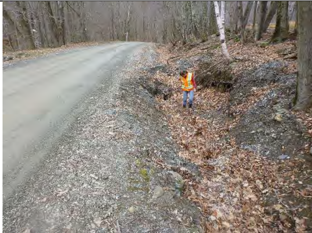
Photo 1: Eroded and unstable ditch upstream of cross-culvert inlet.
