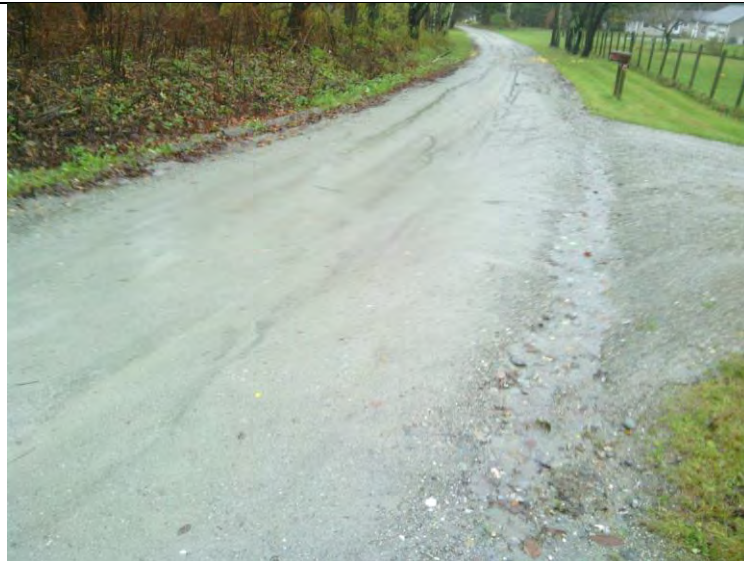
Photo 1: Upper section of Sandgate Road at Woods Gift Lane. Runoff is running along the road edge causing rilling and sedimentation downhill.
