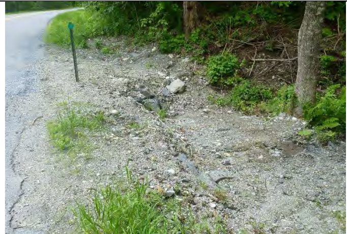
Photo 2: Unstable sediment at a Sandgate Road cross-culvert-inlet.
