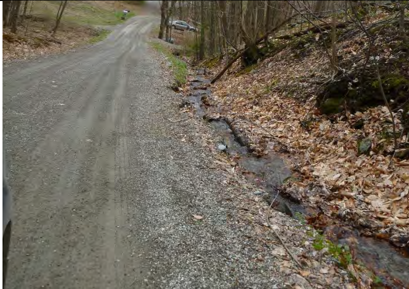
Photo 1: Erosion of steep section of Southeast Corner Road.
