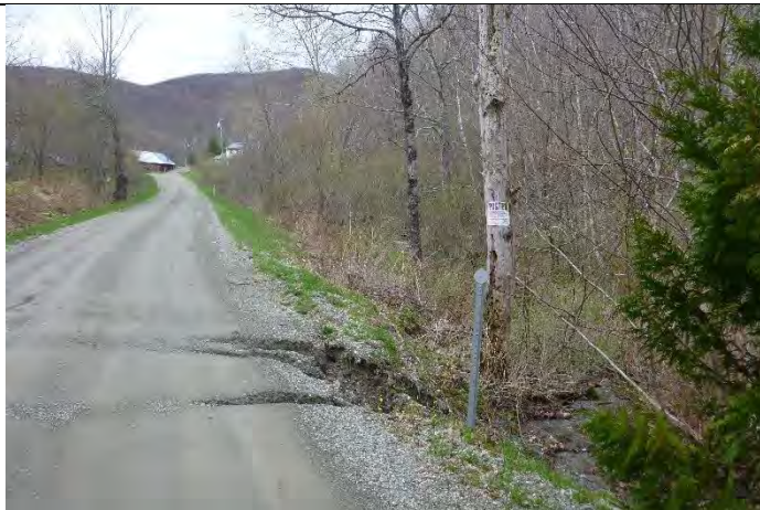
Photo 1: Severe road erosion near a cross-culvert outlet on Wuerslin Road.
