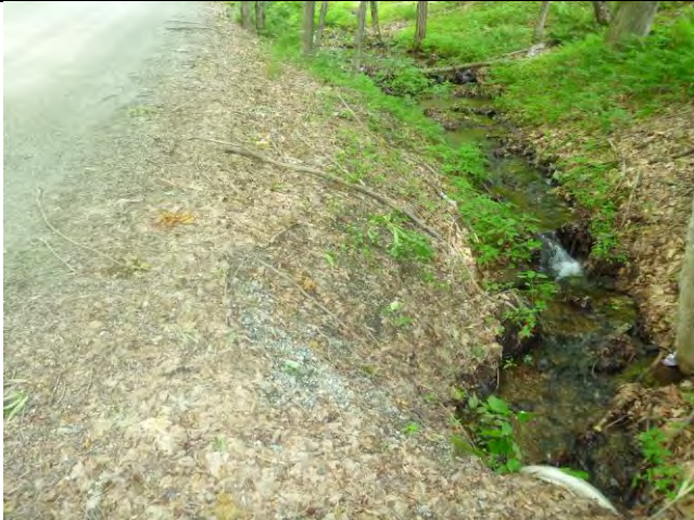
Photo 1: Some bank erosion is present upstream of an undersized culvert on Rupert Road.
