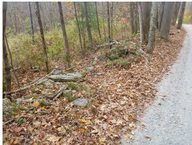
Photo 2: Existing armored turnouts are only partially accessible due to accumulation of road bed material.
