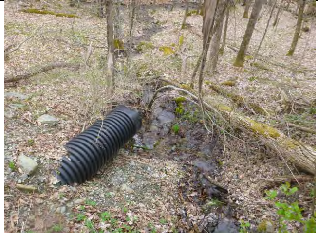
Photo 2: Erosion at the perched outlet of a West Road cross culvert.
