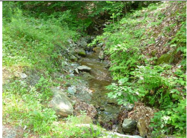
Photo 2: Some bank erosion is present upstream of an undersized culvert on Chunks Brook Road.
