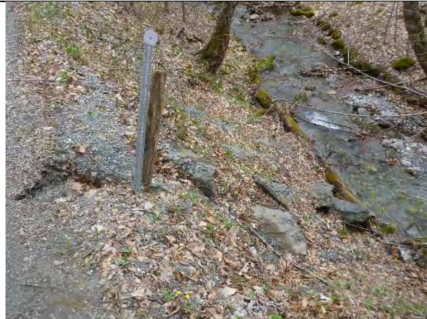
Photo 2: Erosion along the road edge at the cross-culvert outlet adjacent to a second order tributary to the Green River.
