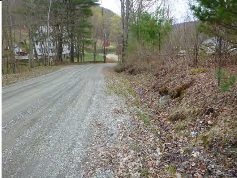
Photo 1: Erosion along a steep section of Southeast Corner Road.
