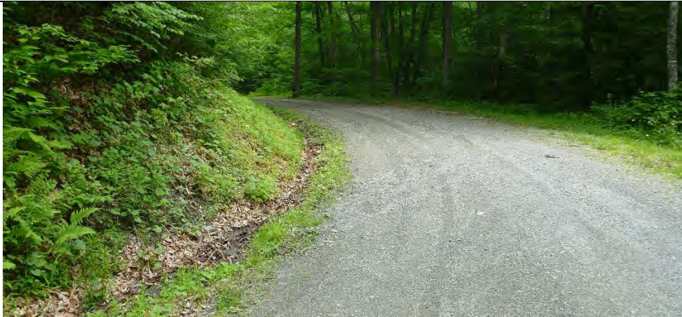
Photo 1: Erosion of steep section of Tate Hill Road.
