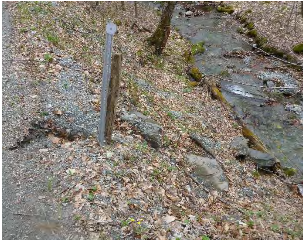
Figure 2: Rilling along the road edge and erosion of the Wilcox Hollow Road cross culvert outfall.
