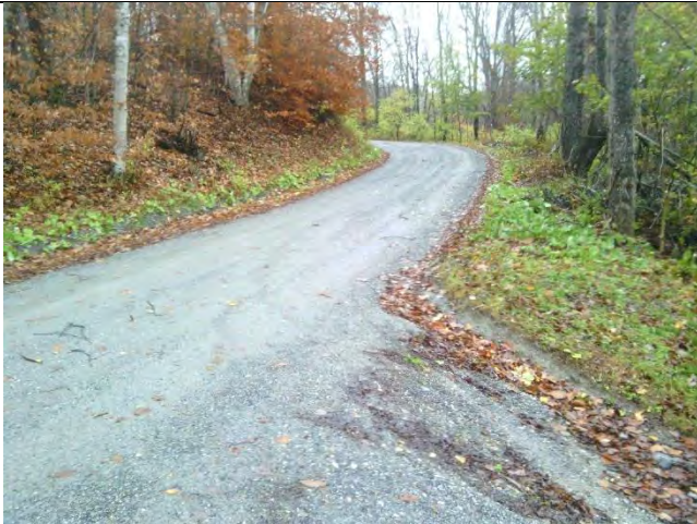
Photo 1: Runoff down a steep portion of Wuerslin Road is causing erosion at the secondary turn to Sandgate Road.
