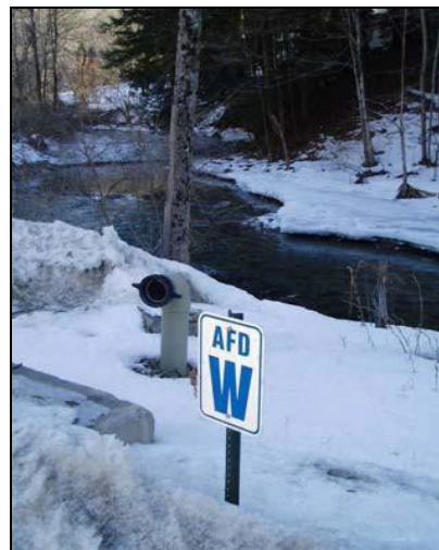
Figure 22: Green River dry hydrant.
