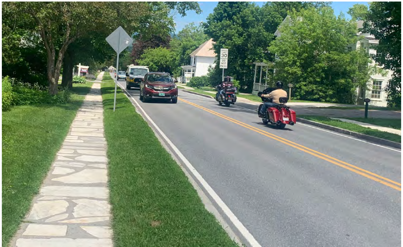
Main St./Route VT 7A has almost no shoulder and a sharp granite curb.
