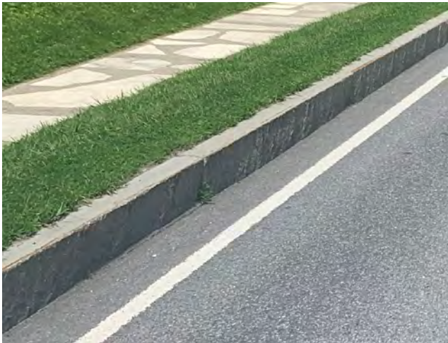
Many survey respondents said the sharp granite curbs on Main St./Route 7A are a hazard to cyclists.
