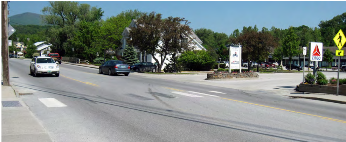
Worn crosswalk, spanning three travel lanes (above). Long crosswalk at Riverside Heights (top right).
