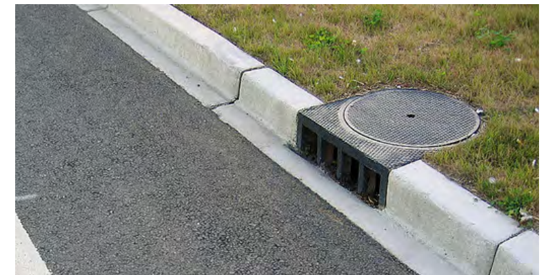
Example of a drain inlet embedded into the face of the curb out of bikes’ way.
