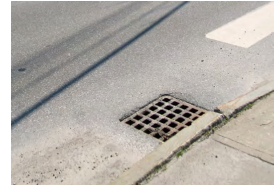
Depot Street's storm grates are a hazard for cyclists.
