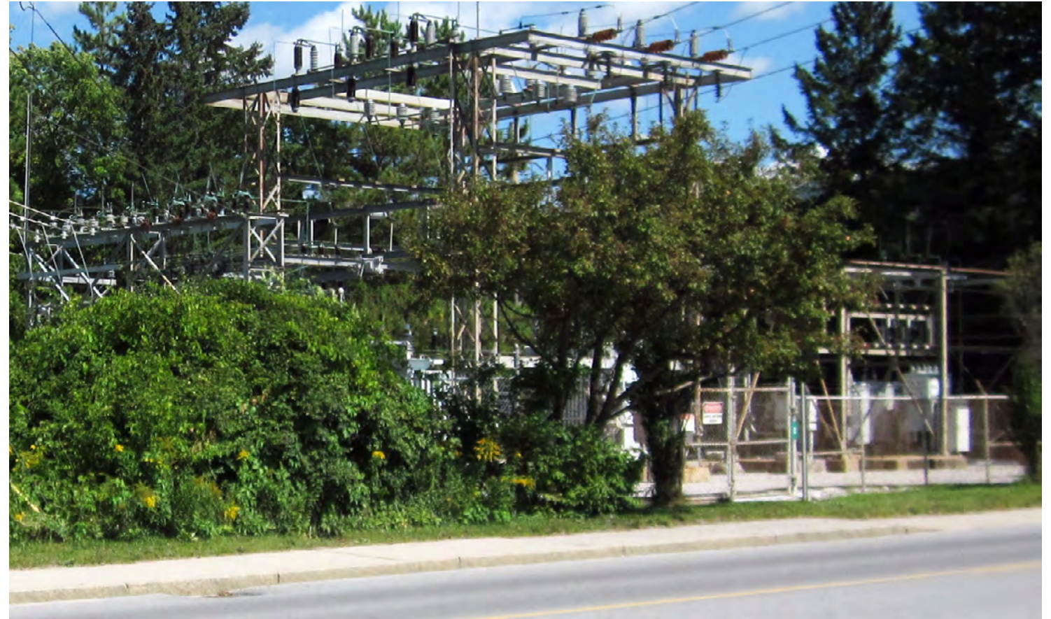
Green Mountain Power's Depot Street substation
