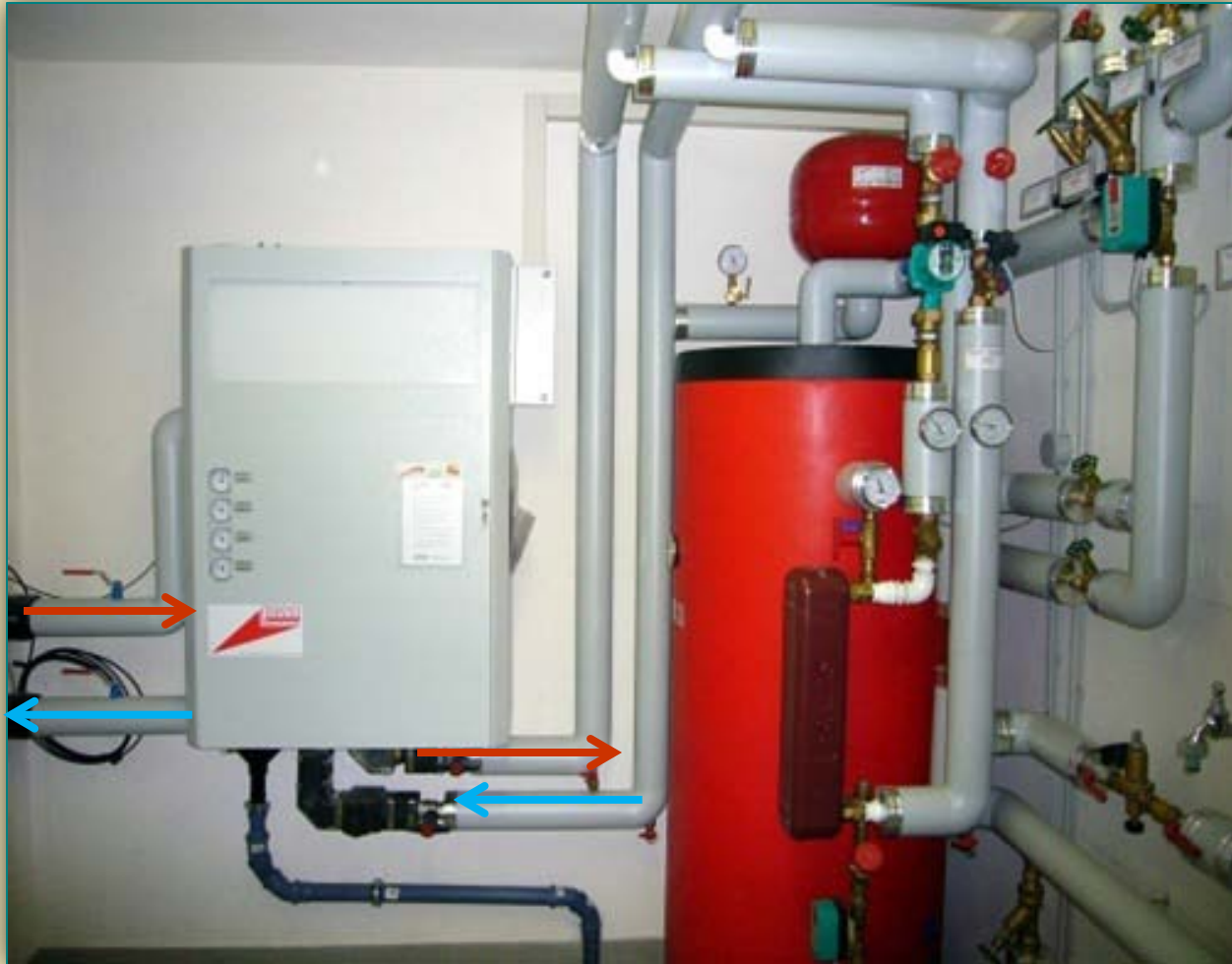
Residential Heat Transfer Station with Metering
