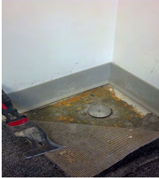
Figure 3: Protective flush mounted cover over the Vapor Pin®
