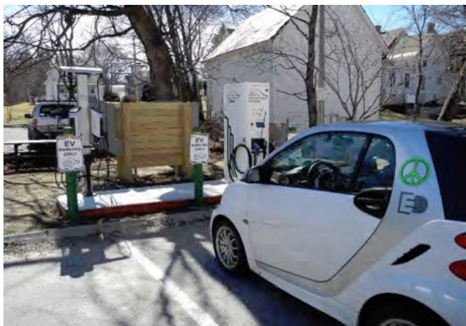
The Town has installed several new high-speed electric vehicle charging stations in municipal parking lots.
