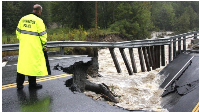
Inspecting the section of the Route 9 bridge east of Bennington that was destroyed during Tropical Storm Irene.
