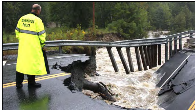
Inspecting the section of the Route 9 bridge east of Bennington that was destroyed during Tropical Storm Irene.
