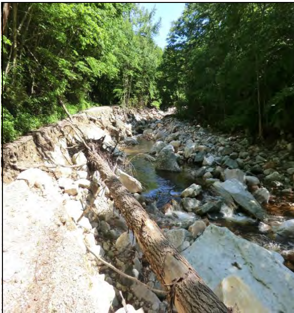
Tropical Storm Irene, in 2011, caused massive damage to the Roaring Branch in Sunderland and to the adjacent Kelley Stand Road (remnant of the road pictured above on the left side of the photograph).
