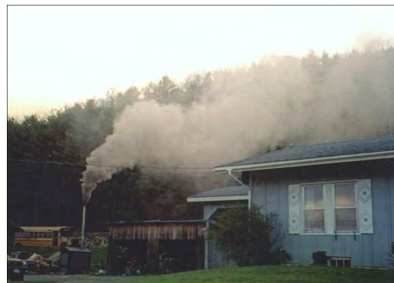
Older outdoor wood-fired boilers can cause serious local air pollution and health effects. A program to promote replacement with cleaner burning is overseen by the Agency of Natural Resources.
