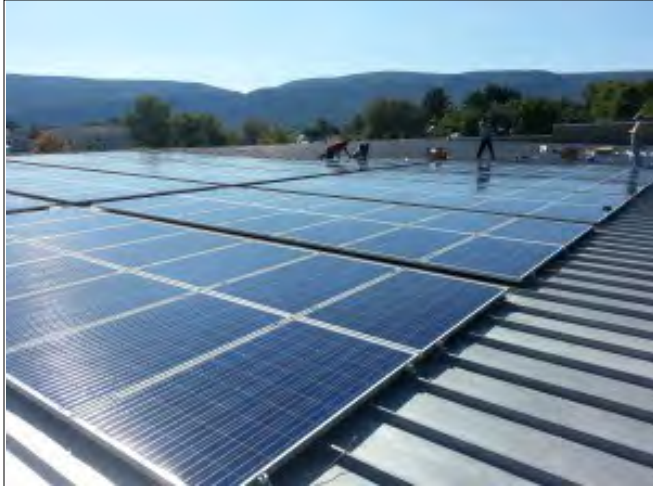
Photovoltaic panels installed on the roof of a building at Hand Motors in Manchester.
