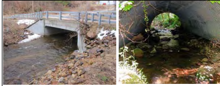
These culverts are large enough to handle flood flows; the depth and speed of water within the culverts provides suitable conditions for movement of stream-dwelling organisms.
