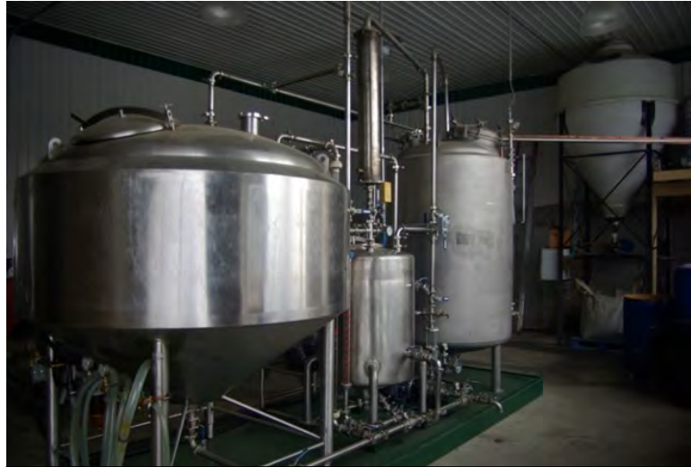
The vegetable oil pressing and biodiesel processing facility at State Line Farm in Shaftsbury demonstrates the potential for liquid biofuels in the region.
