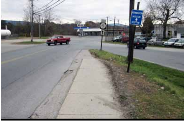
Existing Sidewalks: While there are some existing pedestrian facilities in Segments 1 and 3 of Benmont, they end abruptly in Segment 2.
