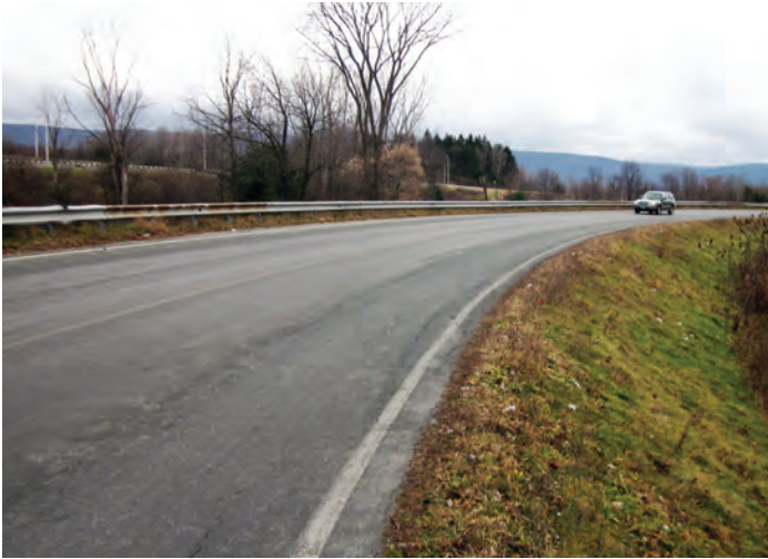
Orchard Road's steep embankments make sidewalk construction unfeasible.
