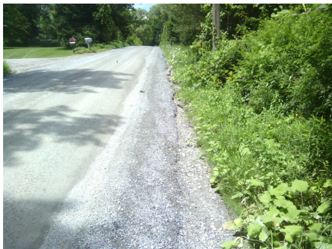
Rill erosion along Tinkham road in Shaftsbury, Vermont.
