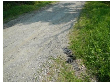
Exposed and damaged culvert.
