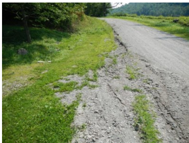
Erosion and deposition along edge of road.
