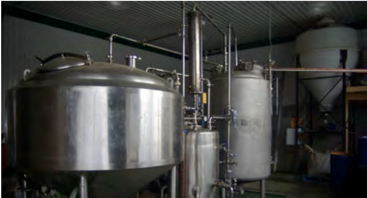
The vegetable oil pressing and biodiesel processing facility at State Line Farm in Shaftsbury demonstrates the potential for liquid biofuels in the region.
