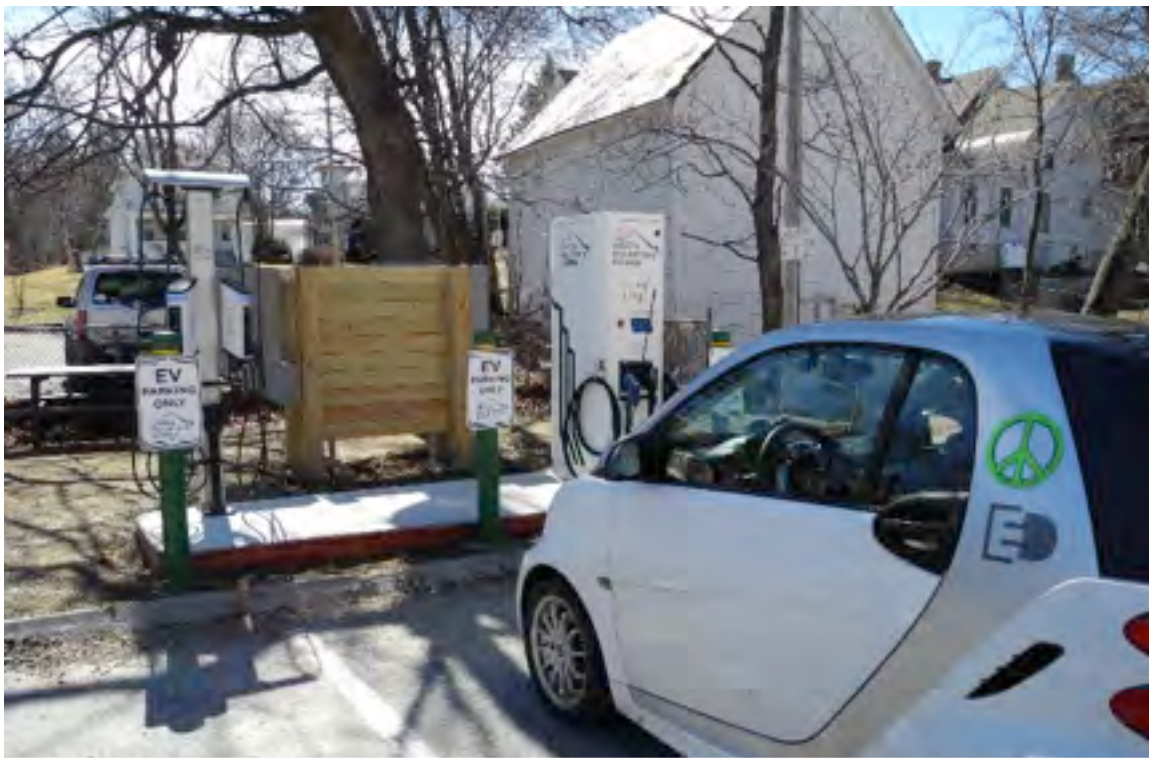
The Town of Bennington has installed several new high-speed electric vehicle charging stations, like this one in downtown Bennington, in municipal parking lots.
