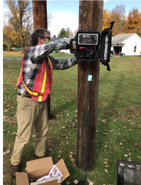
Jim Henderson sets up the BCRC's new radar recorder to collect traffic data on a town road.
