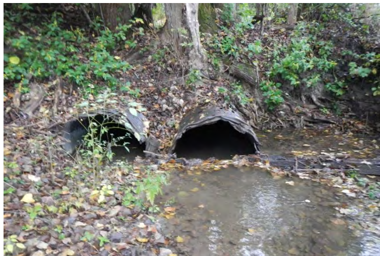
Figure 5.1: Partially plugged undersized culverts on Ladd Brook.
