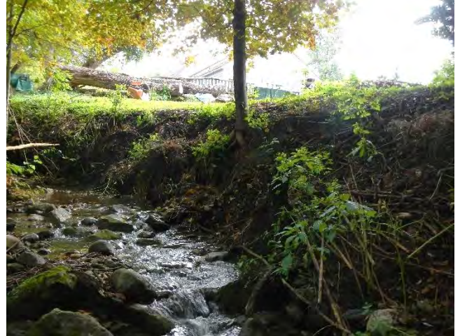
Figure 4.14: Bank erosion and buffer impacts in reach M05S1.01.
